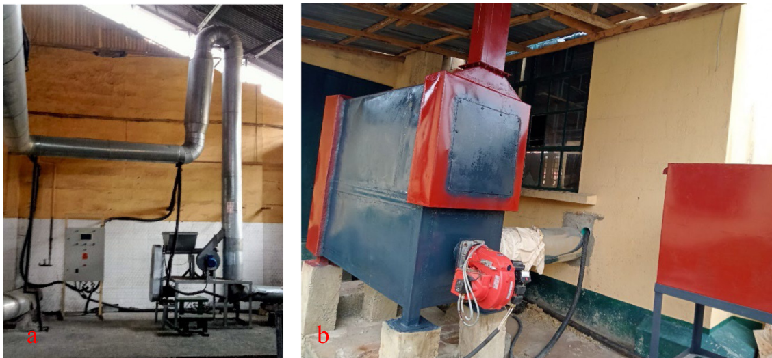
Plate 1. (a): The drying duct with control panel. (b): The heat exchanger with the fuel tank.
