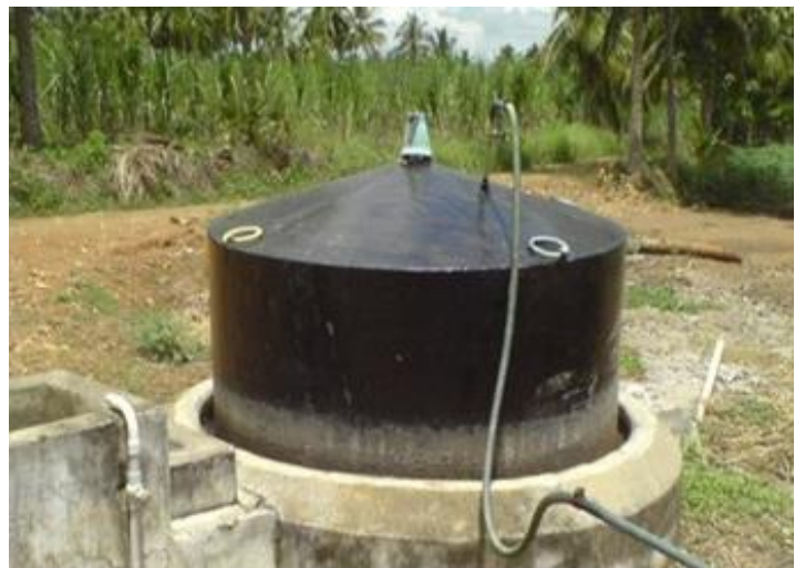
An aboveground biogas reactor; note the pipe used to bleed gasses at the top of the reaction vessel
