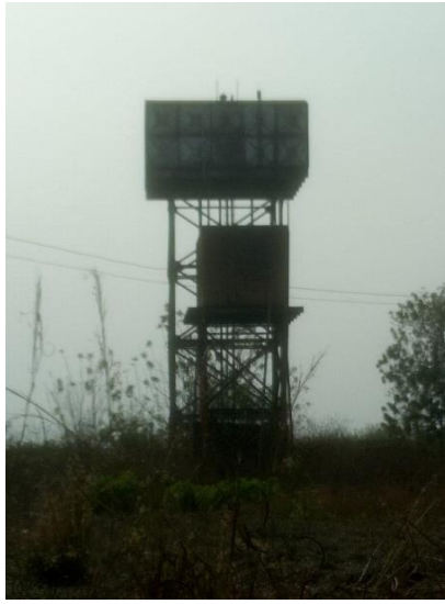
Water storage facility near the entrance of the settlement
