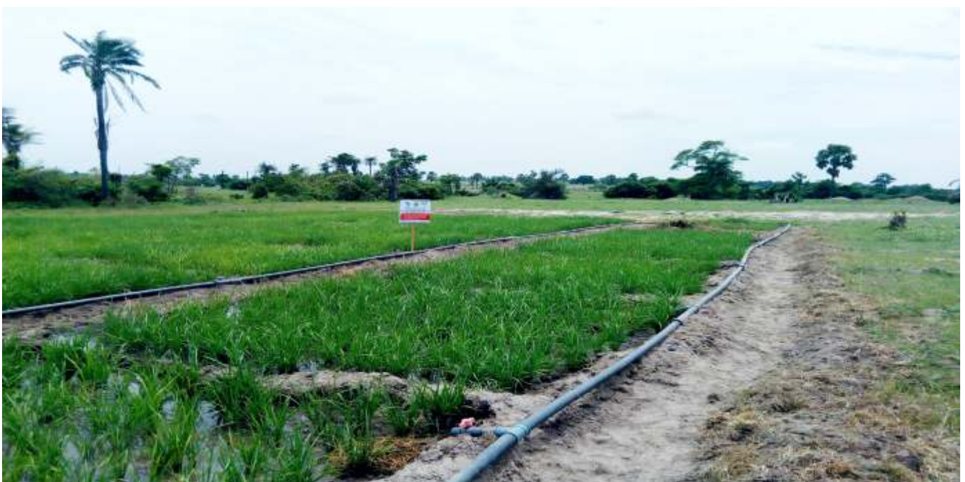
Pressurized PVC pipe distribution system in Nasarawa State, North-Central Nigeria
